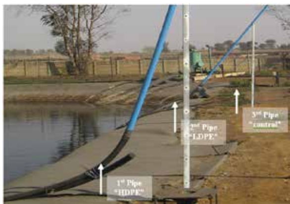
Figure 5: Pipe layout at leachate dam during field tests
