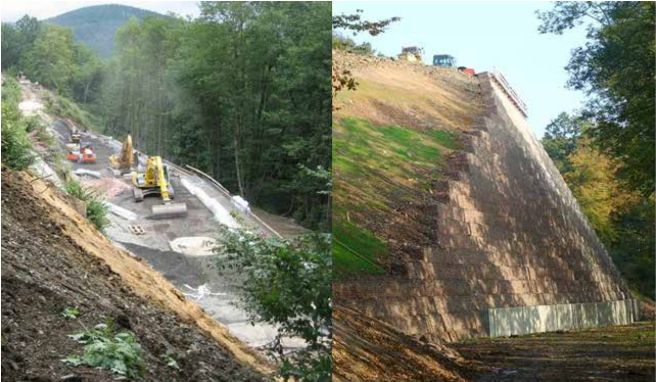
Fig. 7 Retaining structure under construction August 2006 (left) and shortly before completion October 2006 (right)
