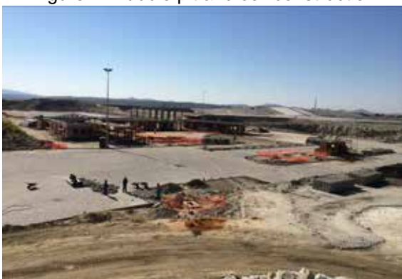
Figure 9: Weigh bridges and offices
