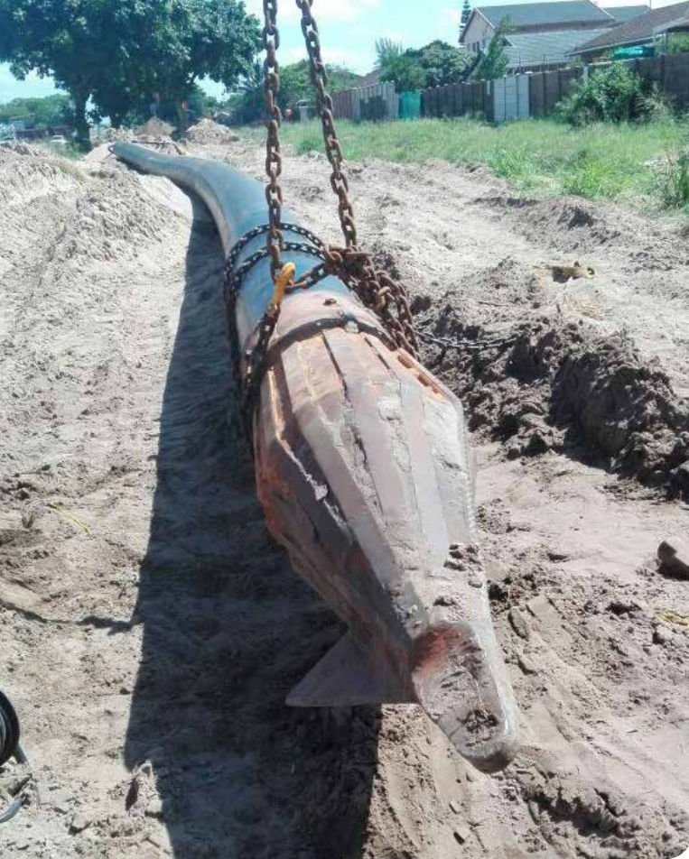
ABOVE RIGHT Pipe splitting of a steel pipe in Barberton ABOVE 450 OD HDPE pipe bursting casing containing a TR 360 hammer
